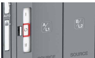
Fig. 3.30 Position of ATS switch is seen from the switch body
