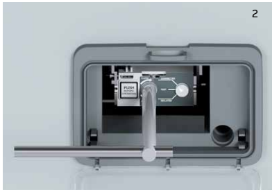
In CONNECTED location, Push button pushed, Racking in/out tool inserted, ready to start rotation
