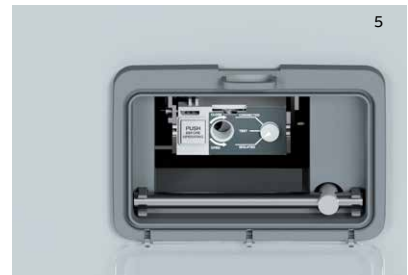
In ISOLATED location, Racking in/out tool inserted back into storage
