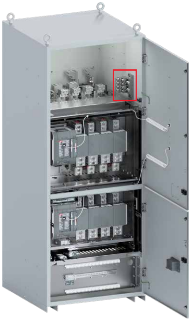
Fig. 7.7 Ground terminal is situated on the top module of Bypass-isolation transfer switch.
