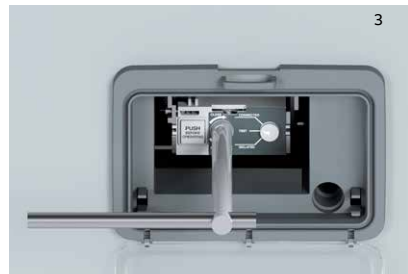
Push button returns, TEST location reached, Push button pushed again, Racking in/out tool inserted, ready to start rotation
